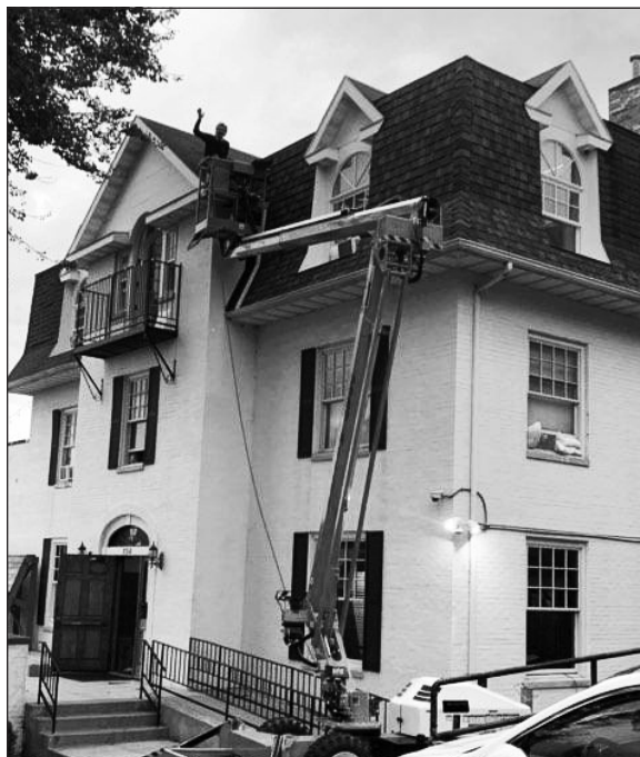
Liviu Rusu '98 on the crane that made it possible to comply with COVID restrictions of working alone. Photo by Mac Ritchie '22.
